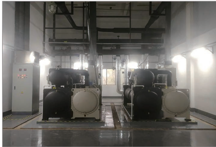
Photo 1 – Elimination and upgrade of lithium bromide units to maglev scroll units in manufacturing center of CRRC Times Electric
