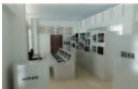
CCTV Monitoring Control Room for the production area
